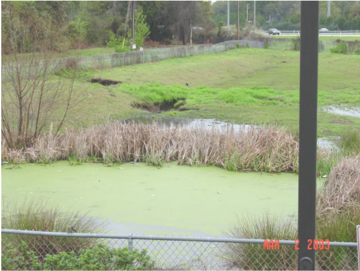
Figure 3. Sinkhole opening in a stormwater basin at northwest corner of Archer Road and I-75. Sinkholes such as this provide a direct link between contaminants in stormwater runoff and the Floridian Aquifer. Repair of such design failures are the responsibility of the basin owner as designated in the original permit.
